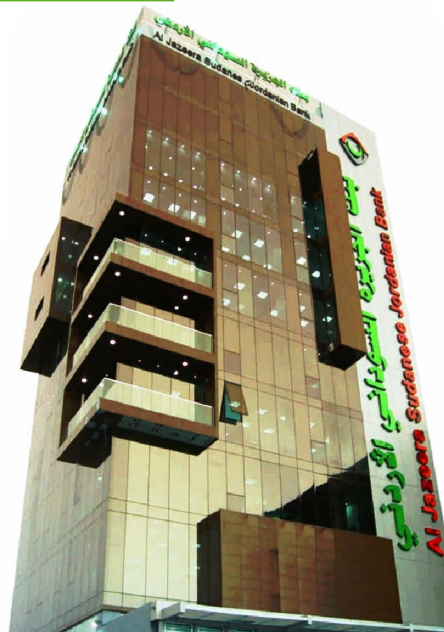
Al-Jazera Sudanese Jordanian Bank (maintenance) .
